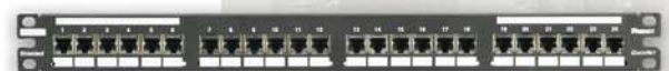
24-port, flat modular patch panel, populated with pre-terminated shielded cassettes with shielded jack modules
